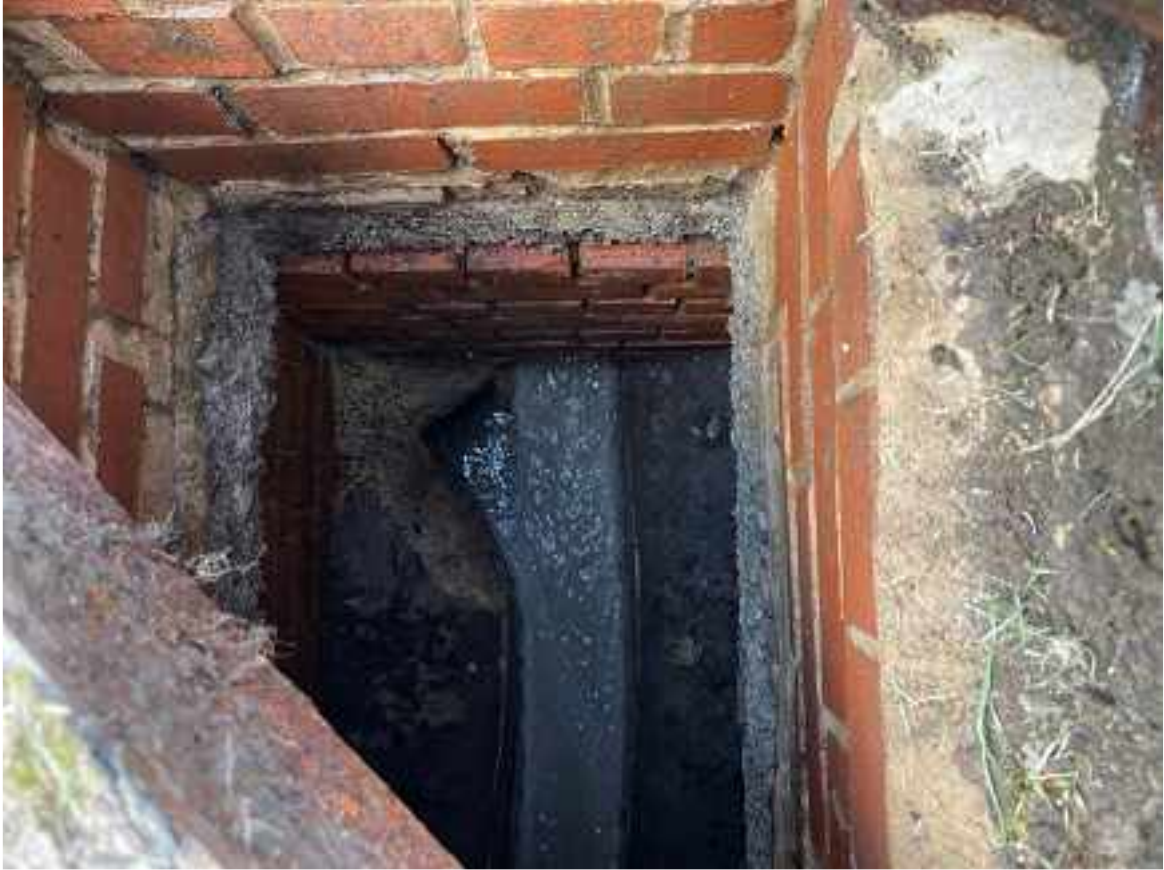
MH 9001 IN ROUNDABOUT
